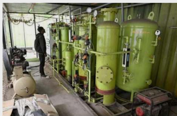
A biogas plant at the Waste-to-Energy unit in Koramangala in Bengaluru. J. ALLEN EGENUSE
