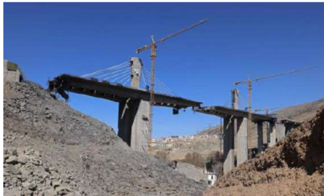
Symbol of resistance: The B1 bridge, after it was destroyed by a strike in Karaj, nearly 35 km southwest of Tehran, on April 3. Donald Trump had previously threatened to bomb Iran 'back to the Stone Ages'. AFP
